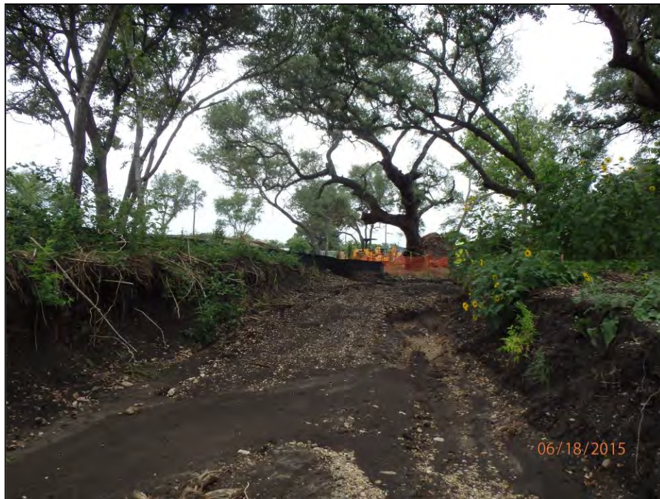
Figure 6-7. Cut bank in northern extent of construction area north of Walnut Branch, facing north.
