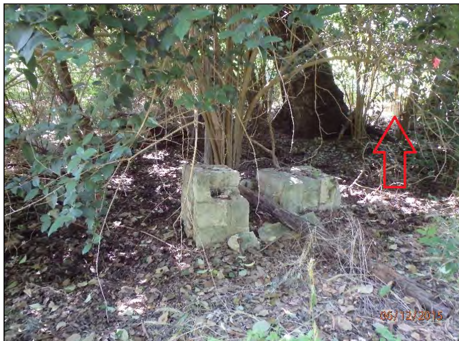
Figure 6-29. Western limestone pillar/gate post (collapsed) with arrow pointing to the outbuilding foundation, facing northwest.
