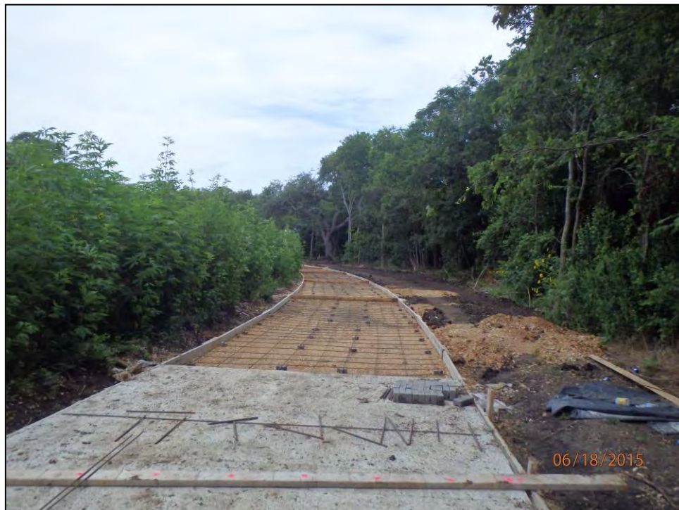
Figure 6-11. Hike and Bike Trail under construction north of Walnut Branch, facing west.
