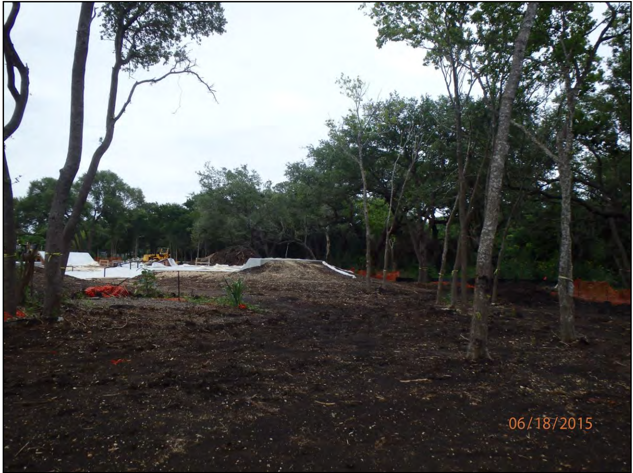
Figure 1-6. Disturbed area south of San Antonio Ave. with the skate park in the background, facing east.
