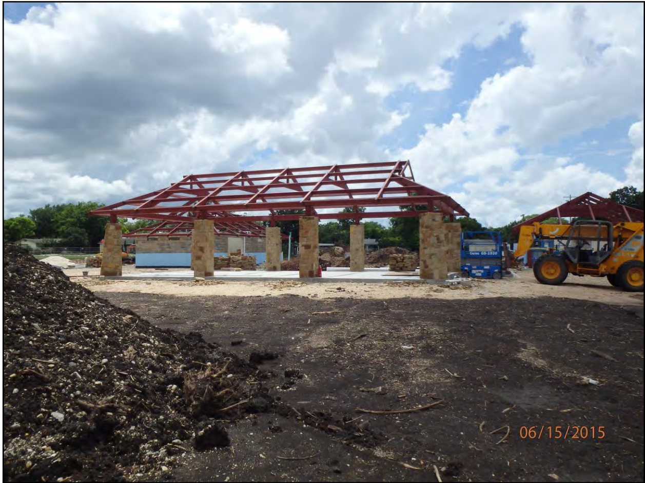
Figure 1-7. Disturbed area east of North Vaughan Ave. showing the restroom (back left), group pavilion (center), and concession building (back right), facing west.
