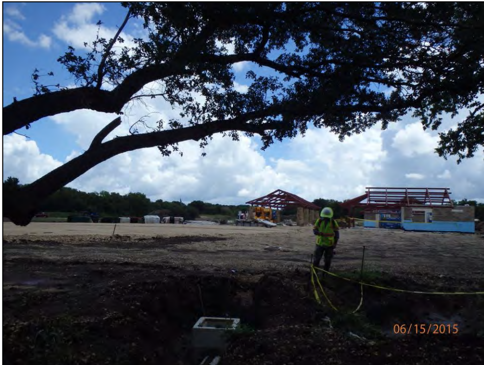
Figure 6-5. Buried culvert in the northern extent of the disturbed area (north central portion of the APE) south of Walnut Branch with concession and group pavilion structures in background, facing south.
