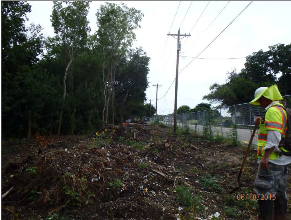
Figure 6-3. Push piles of vegetation and modern trash south of San Antonio Ave., facing west.
