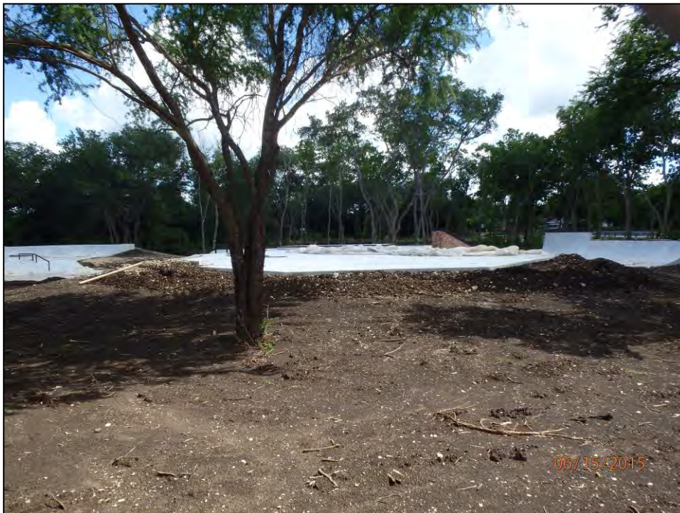
Figure 6-9. Cleared construction area with skate park north of Walnut Branch, facing south.
