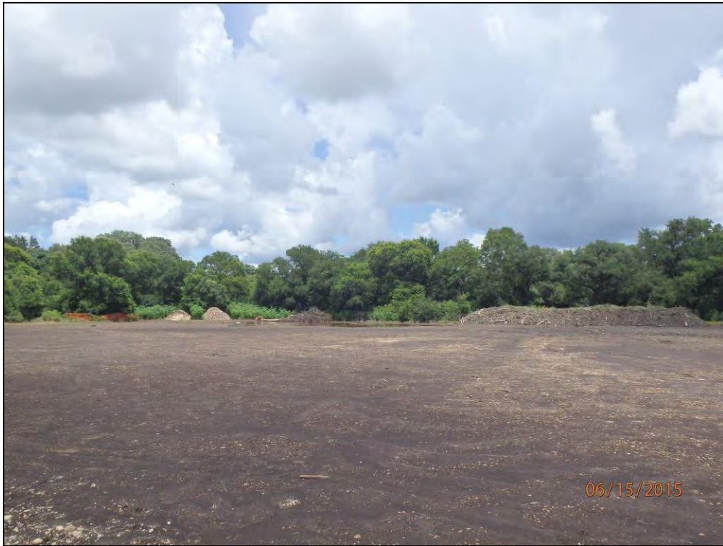
Figure 6-1. Cleared area in the western portion of the APE with push piles, facing west.
