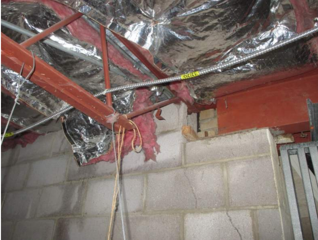
Photo 23: Existing damaged load bearing CMU wall (on east side of the activities/meeting room located west of front entry doors). The steel beam was part of the Addition work, and the joist is part of the original construction. Both the joist and beam have inadequate bearing on the partially removed and cracked CMU. This condition requires structural repair prior to reoccupying the building.
