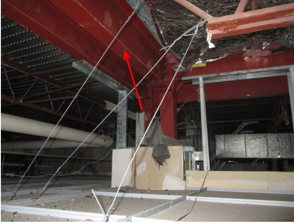
Photo 19: View of expansion joint between original building and addition looking southwest. Roof framing on the left with vented roof deck is part of the Addition. Beam at red arrow was added in 1985 renovation to support existing joists (upper right) and allow removal of a section of original load bearing CMU wall.
