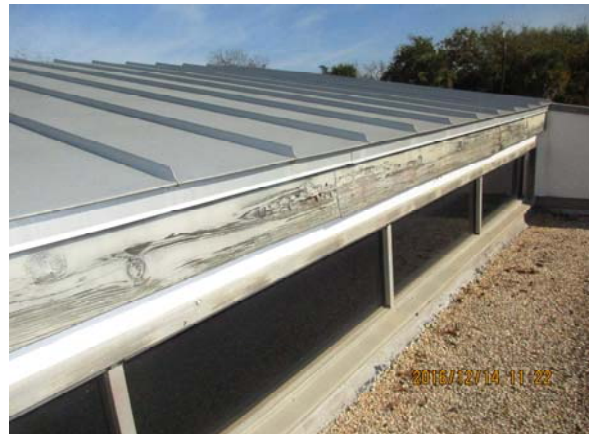
Overview of the metal roof edge and deteriorated wooden fascia.
