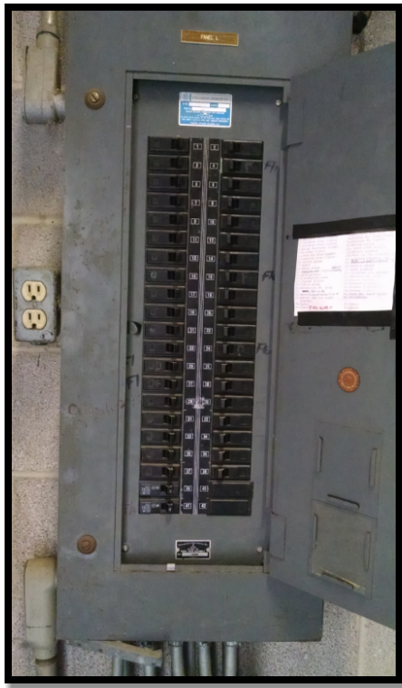
Figure 7 – Electrical Panel “L”
