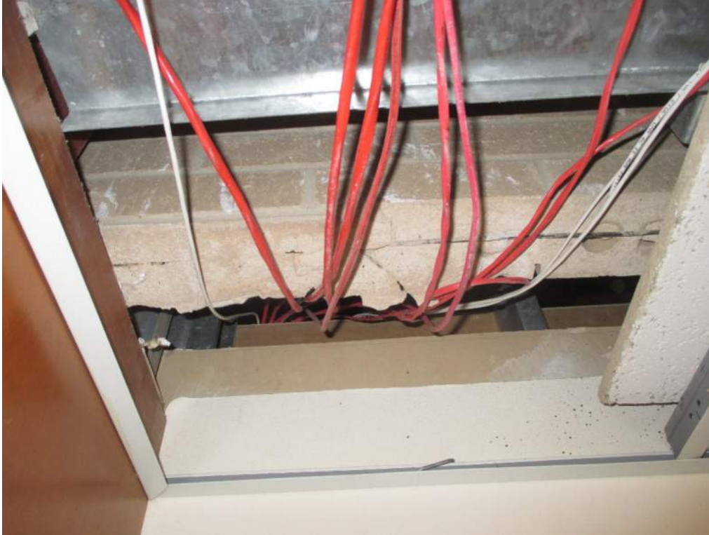
Photo 27: Close-up of unsupported brick veneer above the ceiling at the location of the previous photograph.
