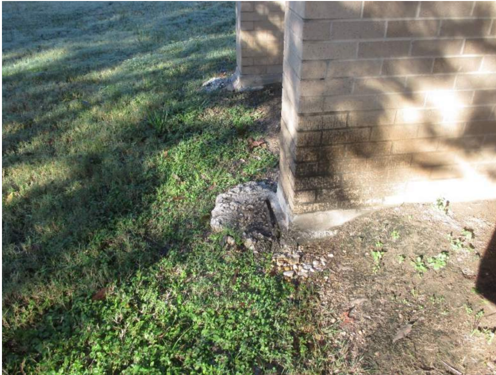
Photo 15: Excess exposed concrete extending beyond formwork line at the foundation for wingwalls on the south side of the addition.
