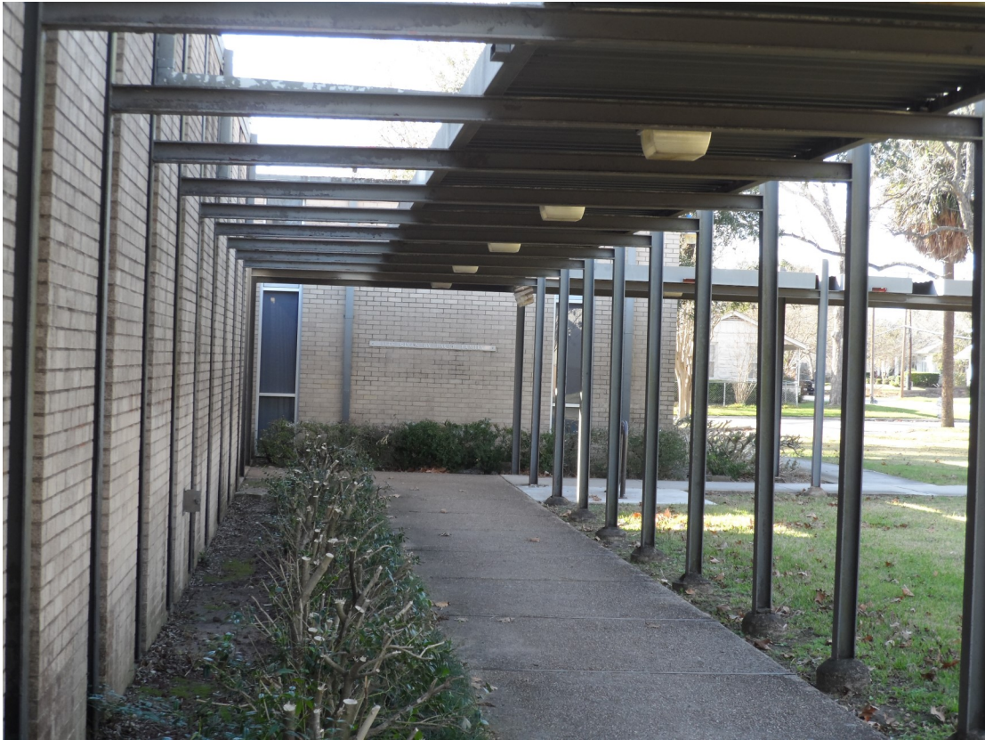
Paint on steel canopy is peeling
