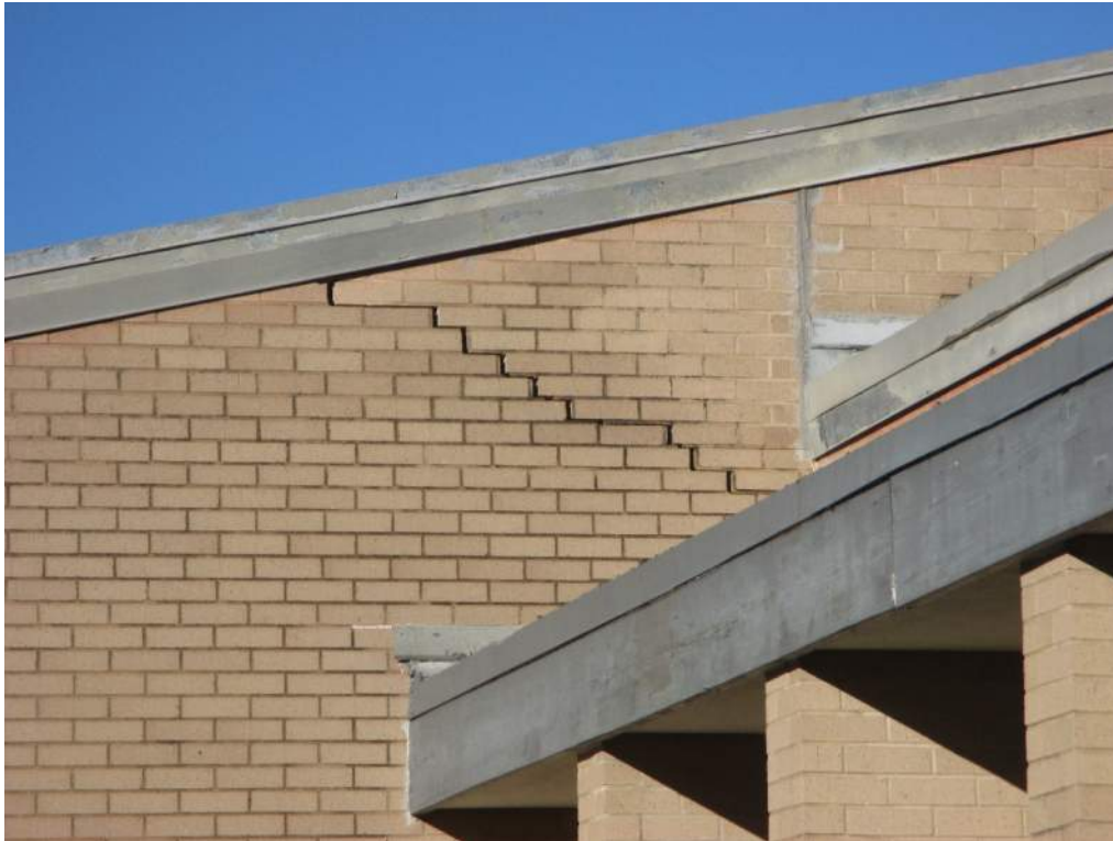
Photo 5: Close-up view of a crack in the brick veneer visible on the east face of the addition where the red arrow occurs in Photo 4.
