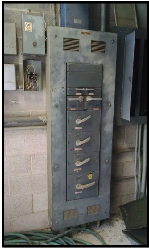
Figure 6 – Electrical Panel "M"
