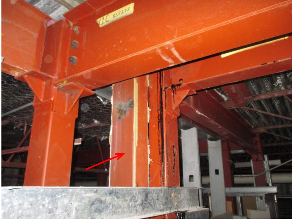
Photo 17: Example of steel roof framing at addition tie-in to existing lobby framing. The existing column at (red arrow) has been supplemented with new columns and framing to create an expansion joint between structures.
