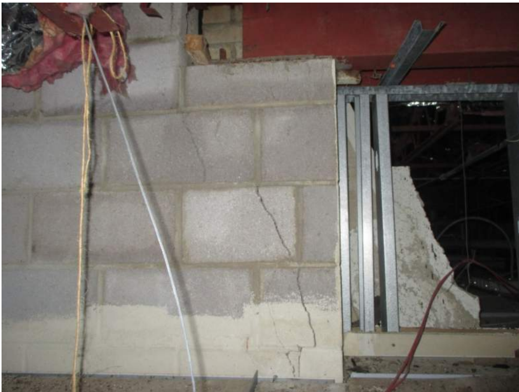
Photo 24: Another view of the cracked load bearing CMU (shown in previous photo) under the steel roof beam.
