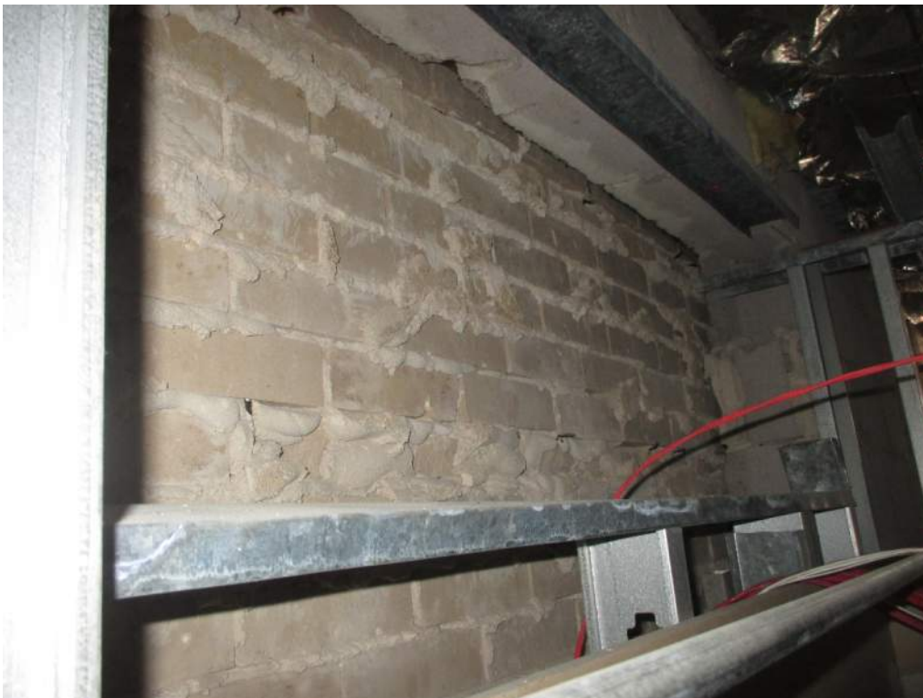
Photo 28: Unsupported brick veneer at the location of the previous photo as viewed looking south from the original building. The existing CMU was removed up to the continuous bond beam at the top of the wall.
