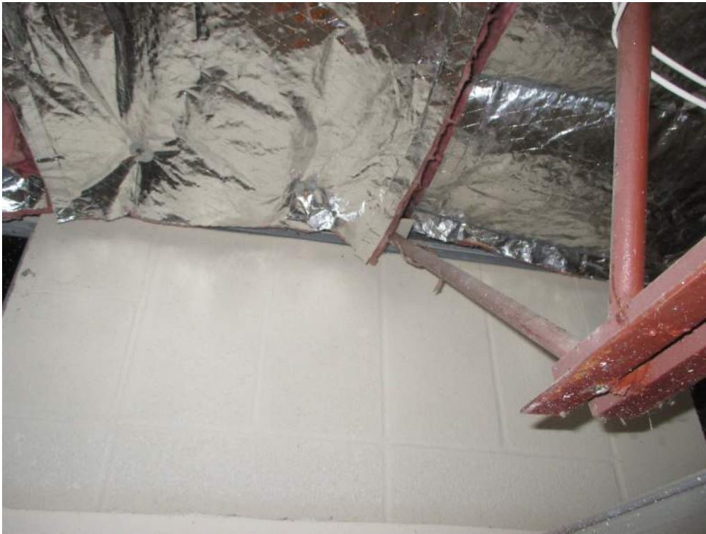
Photo 18: View of a 24" deep open web steel joist bearing on top of load bearing CMU wall in the original Library building. Batt insulation concealed much of the existing roof deck from view in this part of the building.
