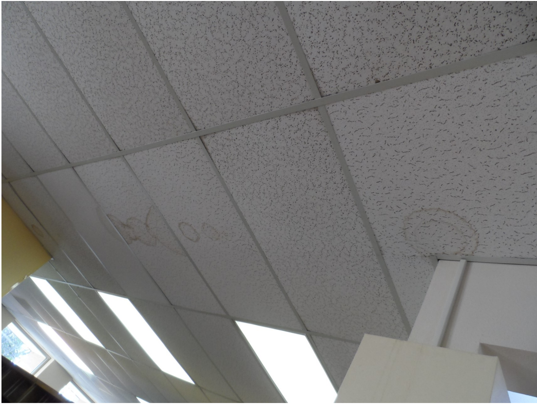
Some acoustical ceiling tiles are stained and many are dirty from age
