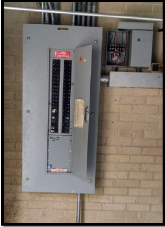
Figure 9 – Electrical Panel “LA”
