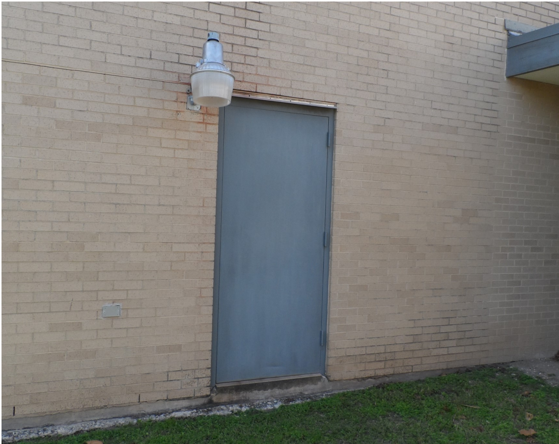
Exterior exit door has a step down to the exterior
