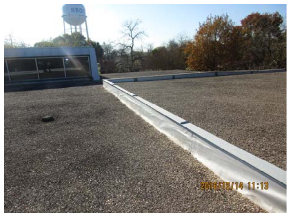
Overview of vertical membrane flashings. Note the wrinkling and delamination of the flashing. Note the expansion joint cover on the joint shown.
