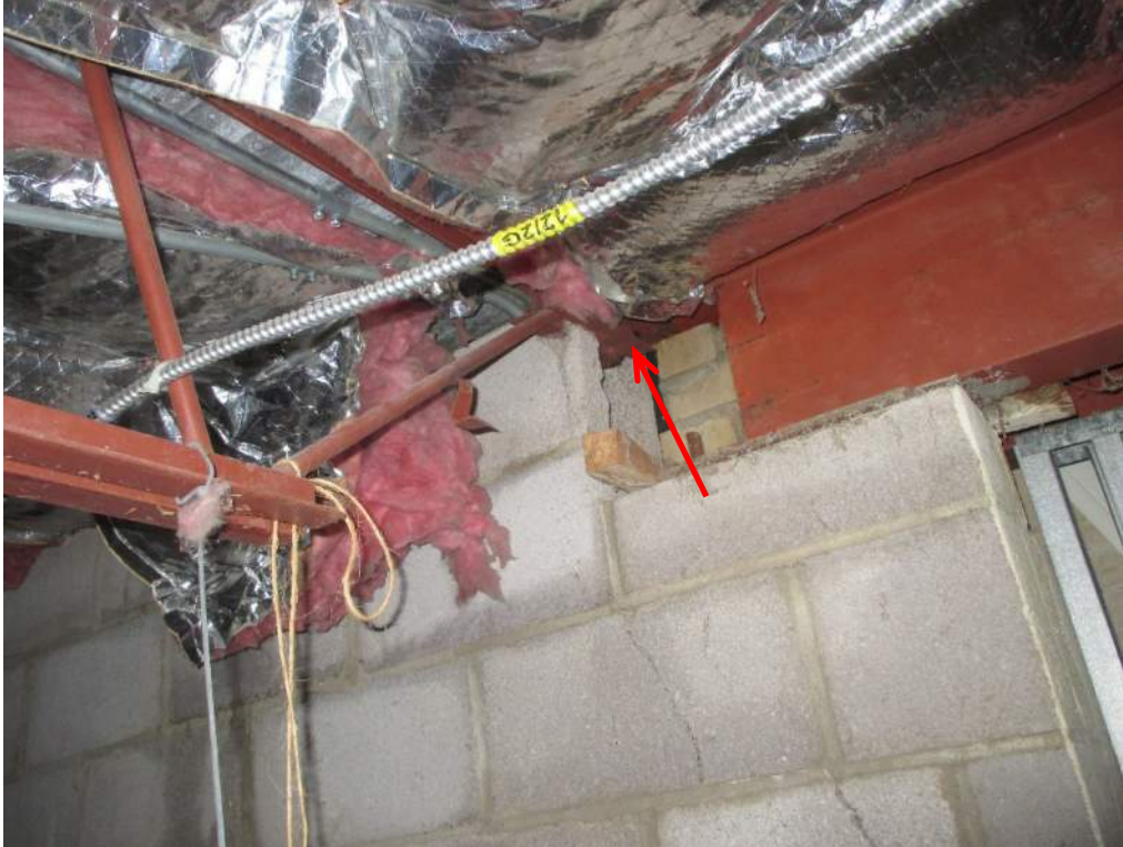
Photo 25: Close-up view of the inadequate joist bearing on the CMU wall. Half of the joist bearing seat no longer has supporting CMU under the seat, and the remaining CMU is cracked.
