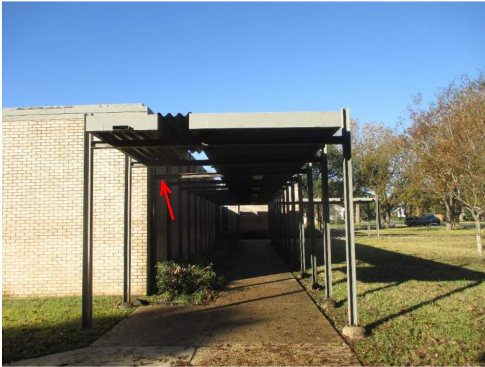
Photo 1: Steel canopy framing at the north (front) side of the building. Individual canopy columns supported by drilled footings were at a visibly different elevation compared to those at building foundation. The canopy roof beam (red arrow) is lower at building side of canopy.
