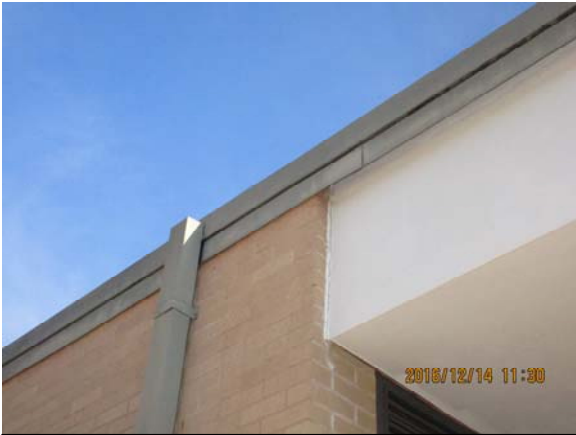
Overview of roof edge guttering. Note the downspout outlet is through the face of the gutter as the gutter is installed on a recessed ledge.
