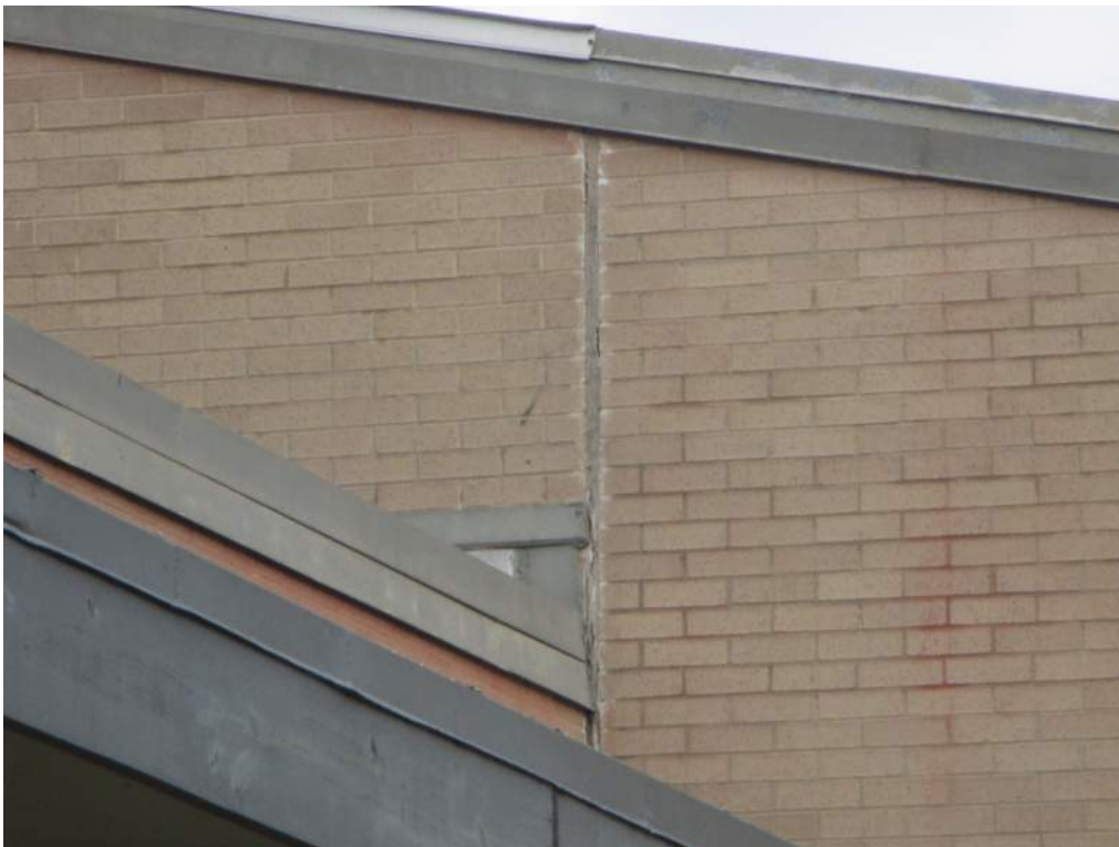
Photo 14: Close-up of cracked sealant in expansion joint shown in previous photograph.
