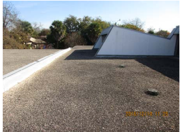
The roof area depicted above include primary roof drains to support drainage. The opening in the background acts as the overflow provision.
