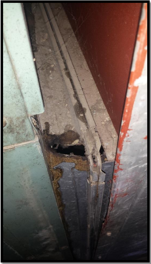
Figure 1 – Ductwork damage on AHU-1
