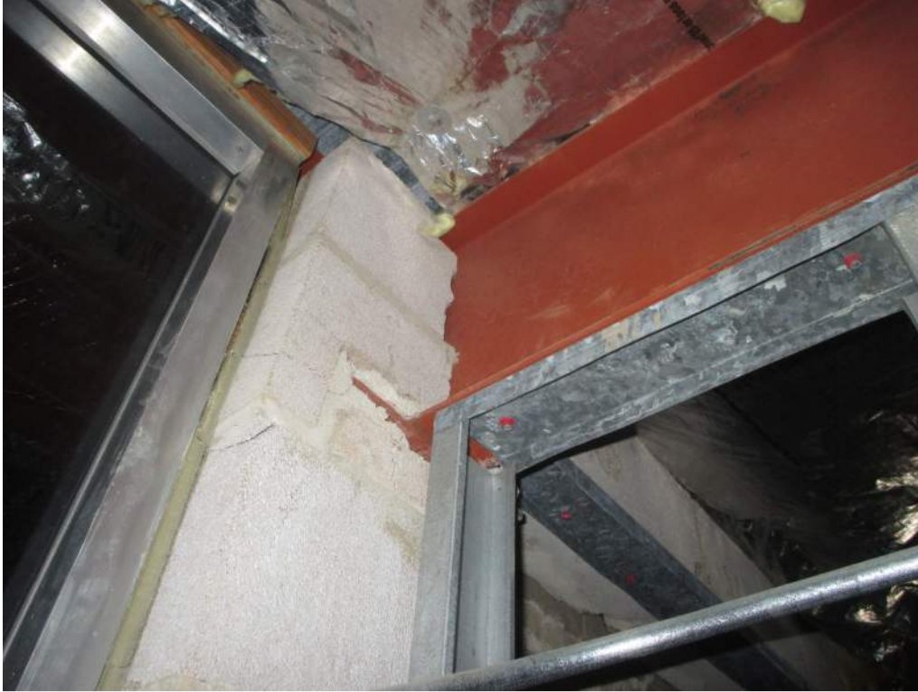
Photo 29: Existing load bearing CMU the was partially removed at the location of the previous photos. An existing original window is visible to the left that was covered over with metal stud wall framing at the Addition. The remaining CMU supporting the beam is cracked and damaged.
