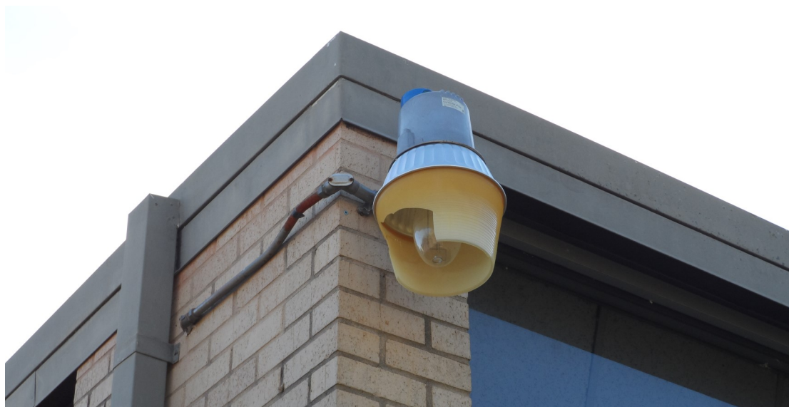
Broken and faded exterior light fixture
