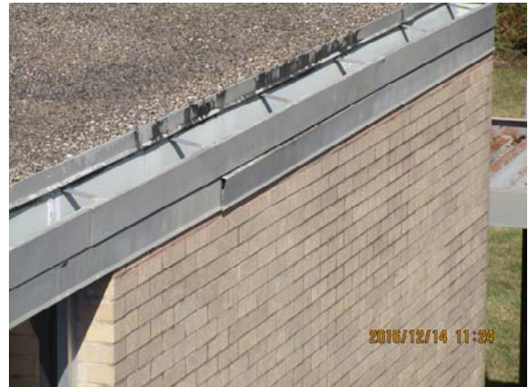
Overview of the low-sloped roof edge. Note the staining of the membrane above the flashing and the open lower flashing joint.
