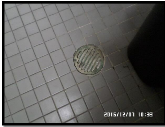
Figure 11 – Blocked Floor Drain
