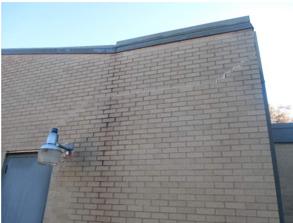
Photo 11: Crack in brick at the southwest corner of the addition.
