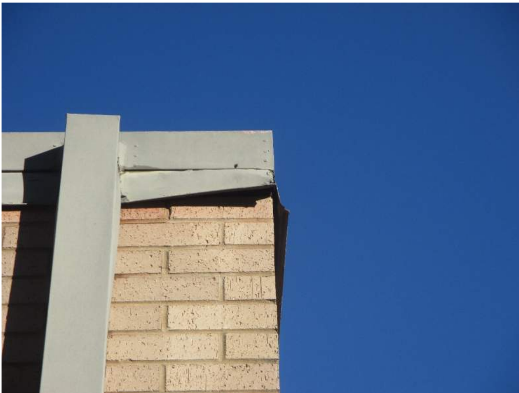
Photo 8: Close-up view of torn sheet metal gravel guard noted in Photo 7 caused by movement of the brick veneer in response to foundation movement.
