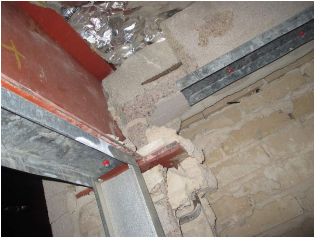
Photo 30: Another view of the end of the partially demolished CMU bond beam, and inadequate bearing for the steel roof beam shown in the previous photo. This condition requires structural repair prior to reoccupying the building.
