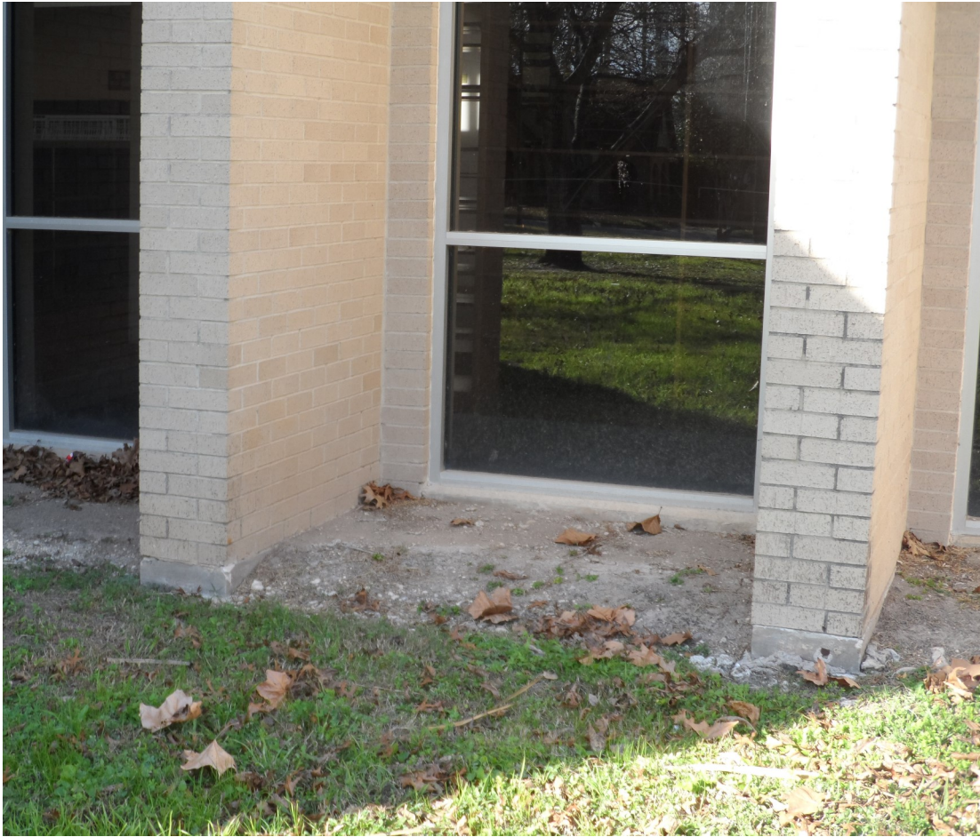
Exposed foundation at masonry fins on South façade eroding
