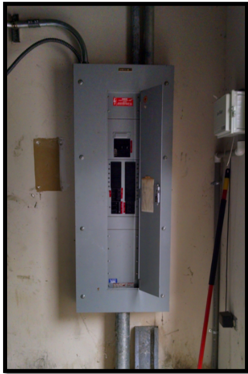
Figure 8 – Electrical Panel “A”
