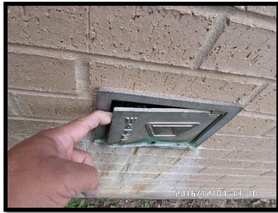
Figure 12 – Damaged Wall Hydrant
