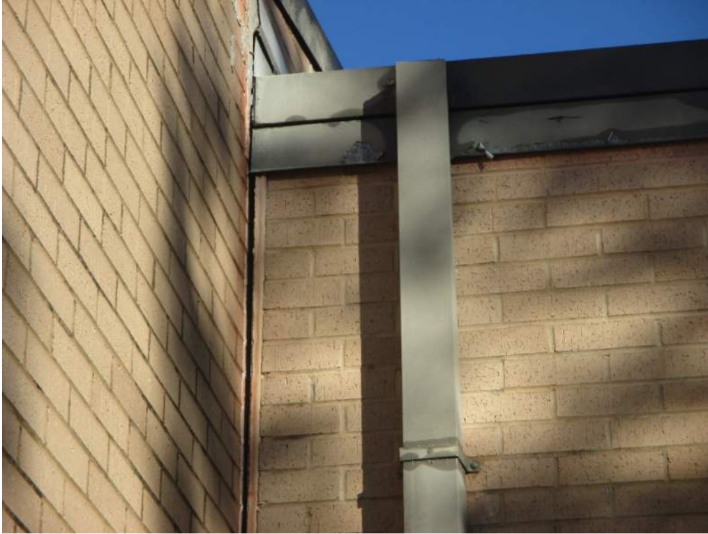
Photo 9: Separated sealant joint caused by foundation movement at re-entrant corner on south side of building.
