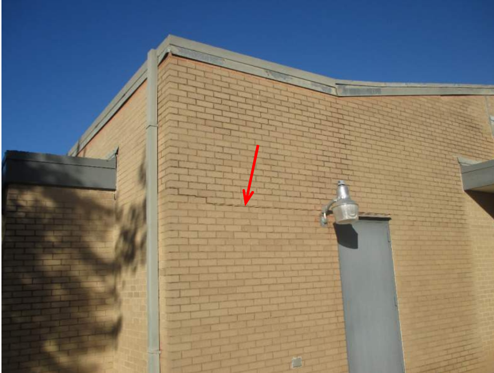
Photo 7: Horizontal crack in brick at top of door frame on east wall of addition. The cracked brick in Photo 5 is at the right side of this Photo. Note the torn sheet metal gravel guard at the top of the brick.
