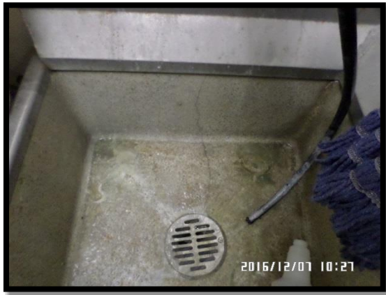
Figure 10 – Cracked Mop Basin
