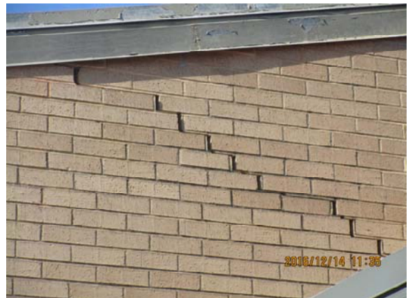
Cracking at an exterior brick veneer wall.
