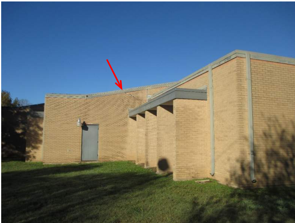
Photo 4: Southeast corner of the 1985 Addition where the exterior wall slopes up to match the sloping roof at the three clerestory skylights constructed in the Addition roof. Also, see Photo 5 for crack in brick at this location.
