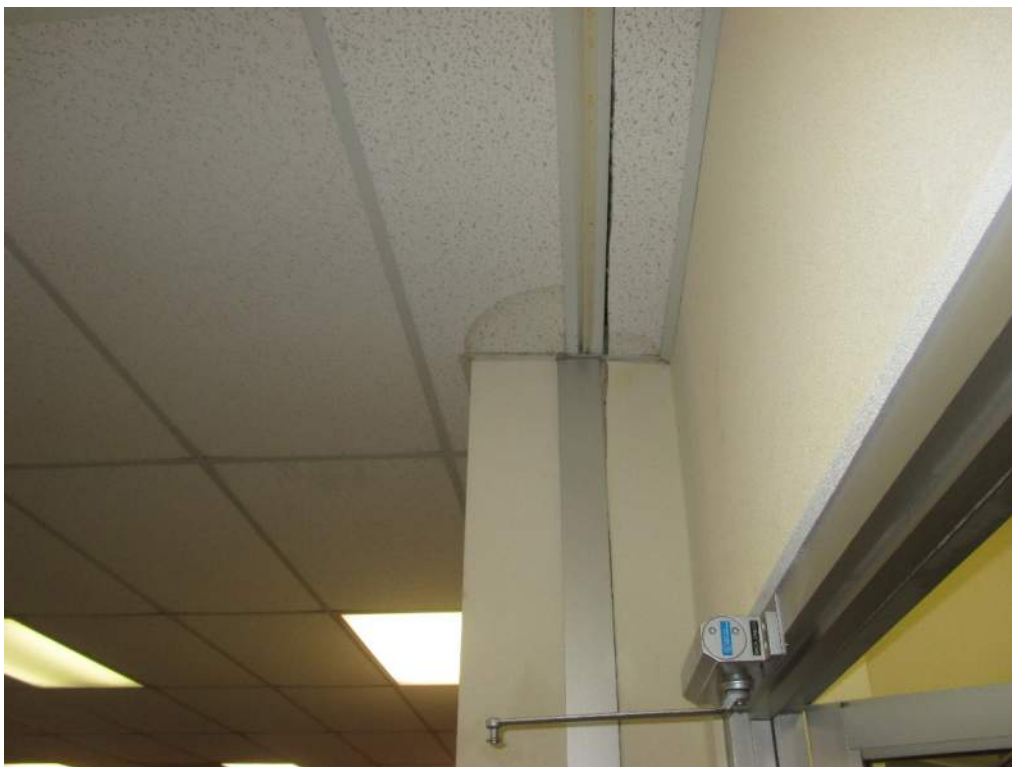
Photo 22: Ceiling expansion joint between the original building and new addition. Evidence of movement, and water staining on the ceiling.
