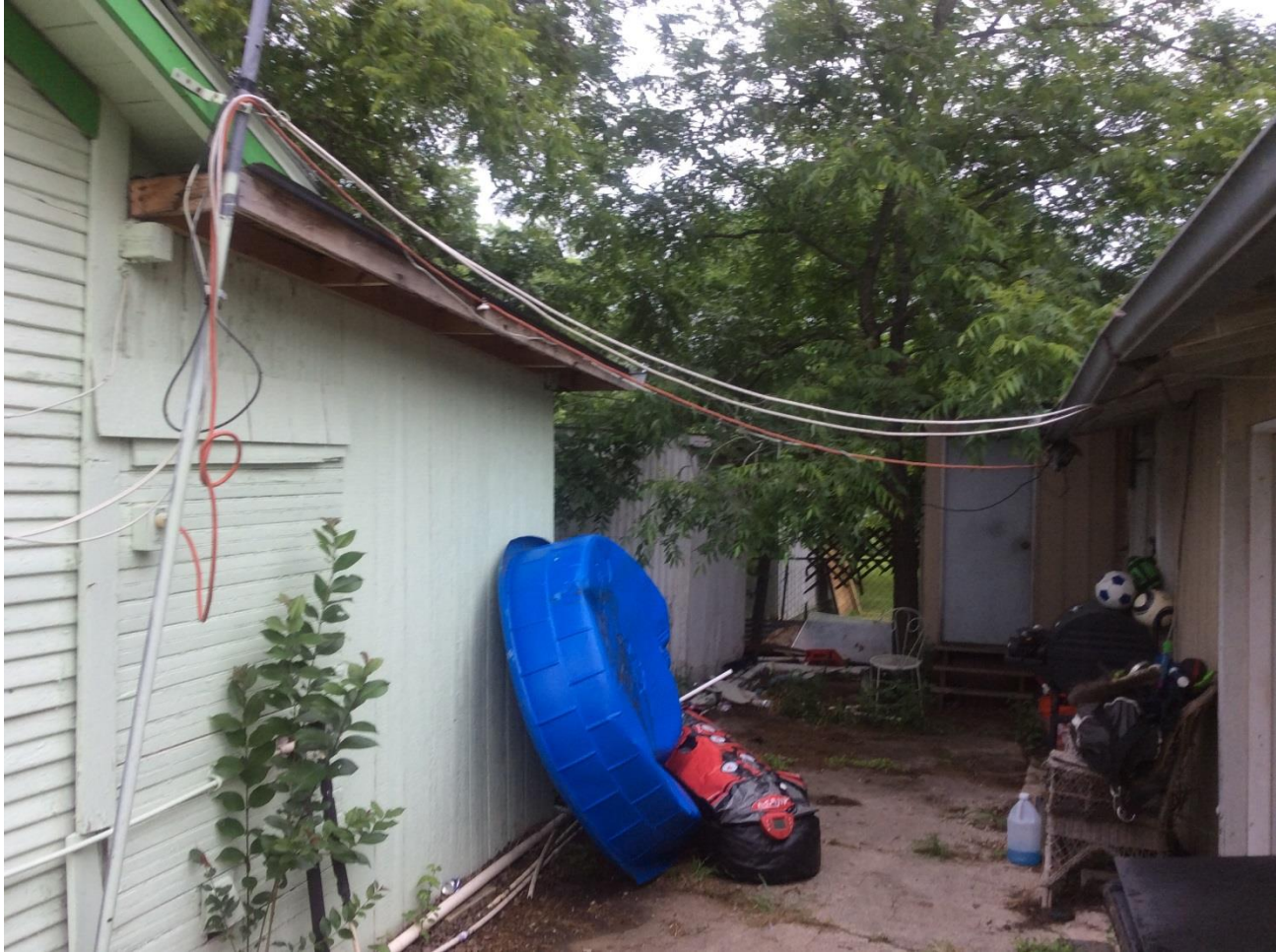
No utilities – extension cords to accessory structures
