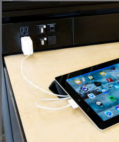
convenience power & data
