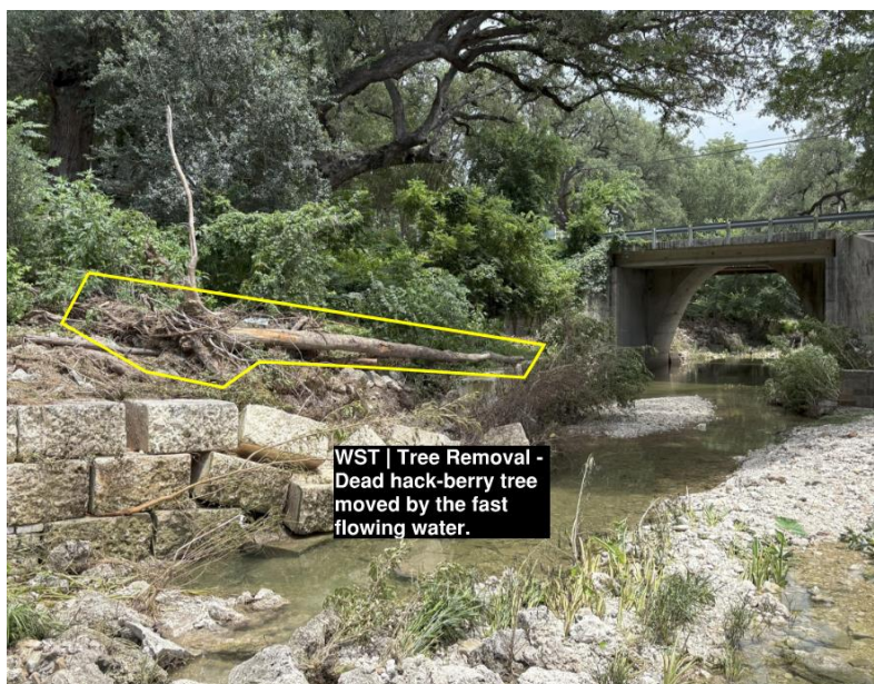
Figure 2: Damage due to July 5, 2025 flood event
