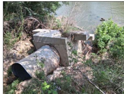
DISCONNECTED OUTFALL STRUCTURE AND SEDIMENT (MAY HAVE EXPANDED SINCE PHOTO)
