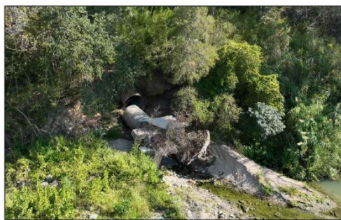
DISCONNECTED OUTFALL STRUCTURE AND SEDIMENT TO BE REMOVED
