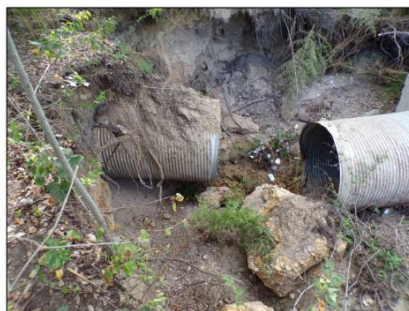
DISCONNECT OUTFALL STRUCTURE AND SCOUR HOLE (MAY HAVE EXPANDED SINCE PHOTO)
